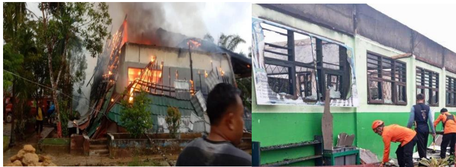
Figure 1. Post-fire condition of SDN 022 Penajam on January 31, 2024, showing partial destruction of the school building (photo: field documentation)
