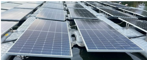
Fig. 1 A 100kWp FPV in Muara Nusa Dua Reservoir, Bali
